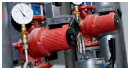
Actuators, valves, control cabinets
